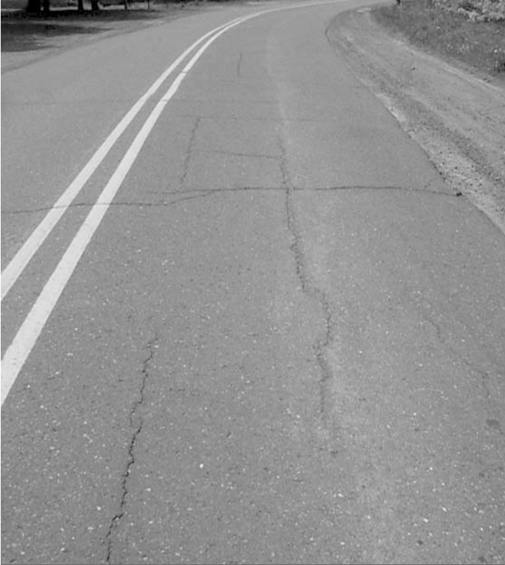
Figure 2.3 - Example of medium density cracking
