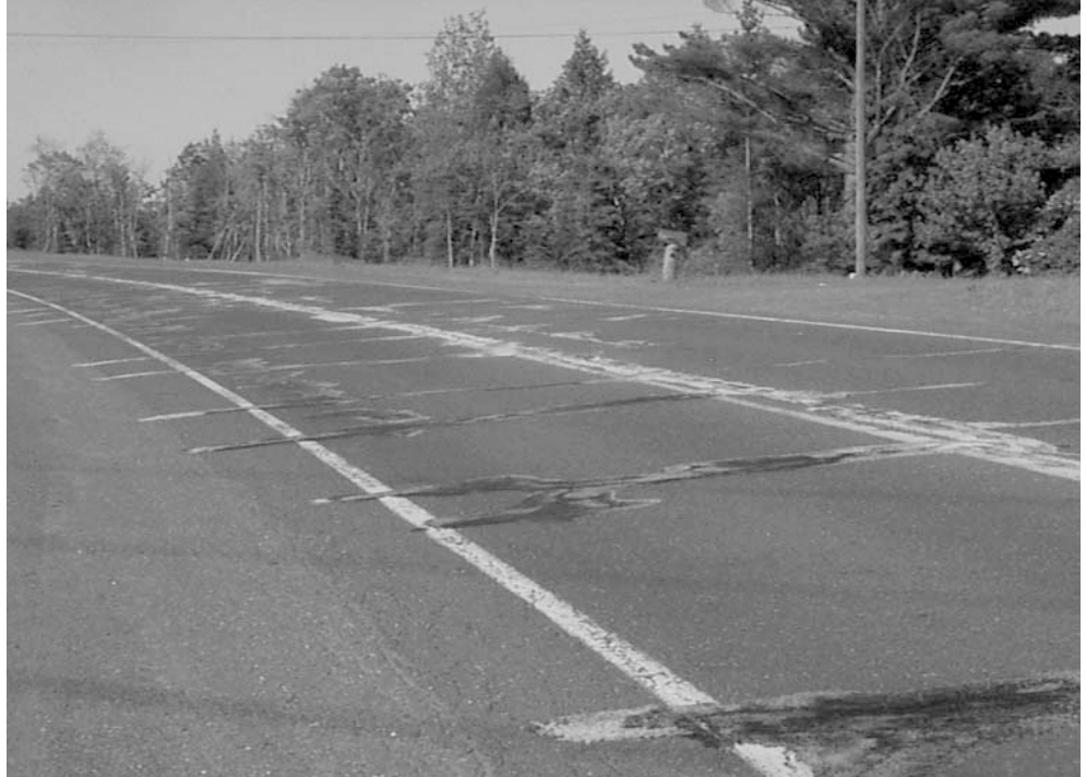
Figure 2.5 - Example of high density cracking
