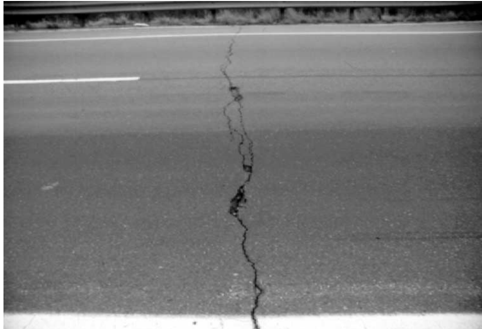
Figure 1. 2 - AC pavement crack suitable for filling
