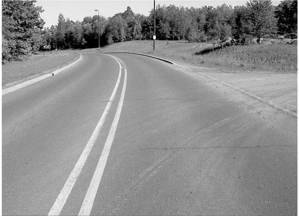
Figure 2.1 - Example of low density cracking
