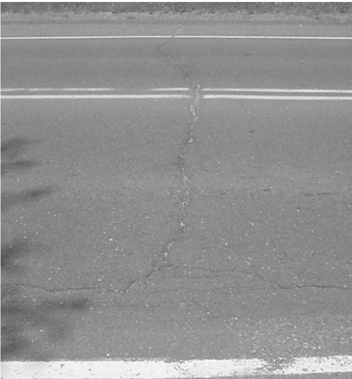
Figure 2.4 - Example of cracking with medium edge deterioration
