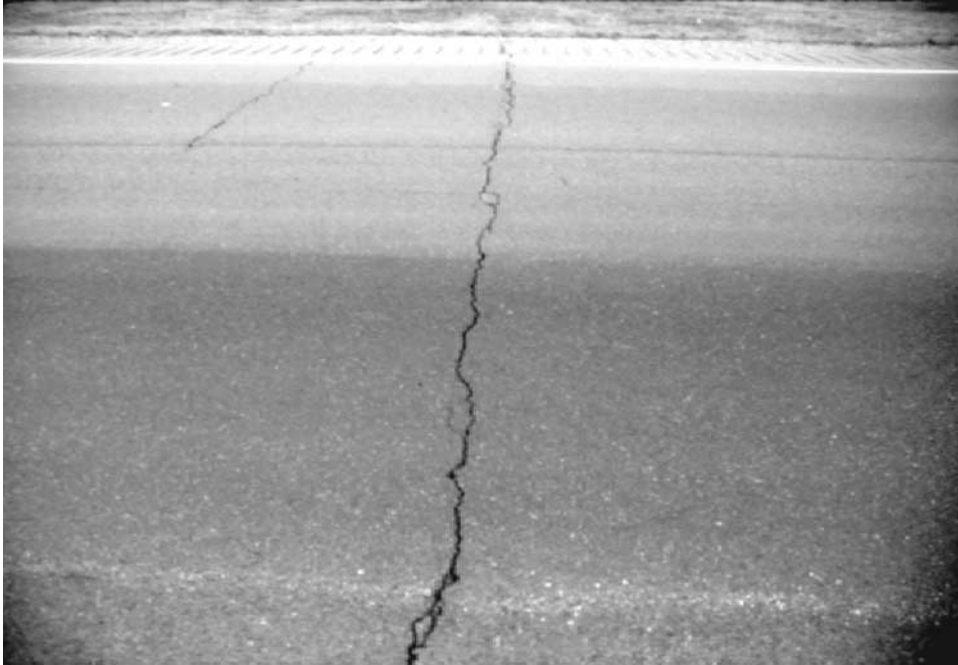
Figure 1.1 - AC pavement crack suitable for sealing
